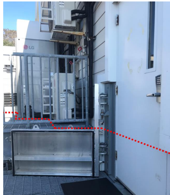
Elevated first floor, elevated systems, and door flood barrier up to design flood elevation at USCG Woods Hole
