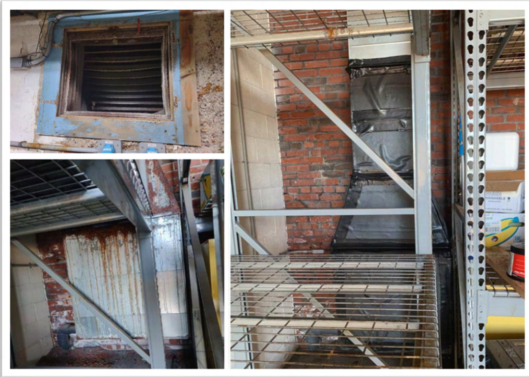
Figure 5. The aquarium basement ventilation system before floodproofing measures (left top and bottom pictures) and after floodproofing measures were implemented (right picture).
