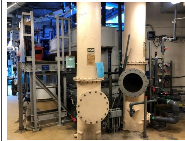
Figure 7: The current life support system for the proposed Super Coral exhibit will need to be upgraded.
