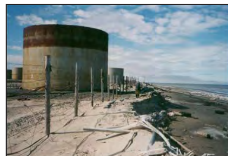
Figure 18: Wave-cut cliff near the Varandei oil terminal, Perchora Sea (Ogorodov 2005).
